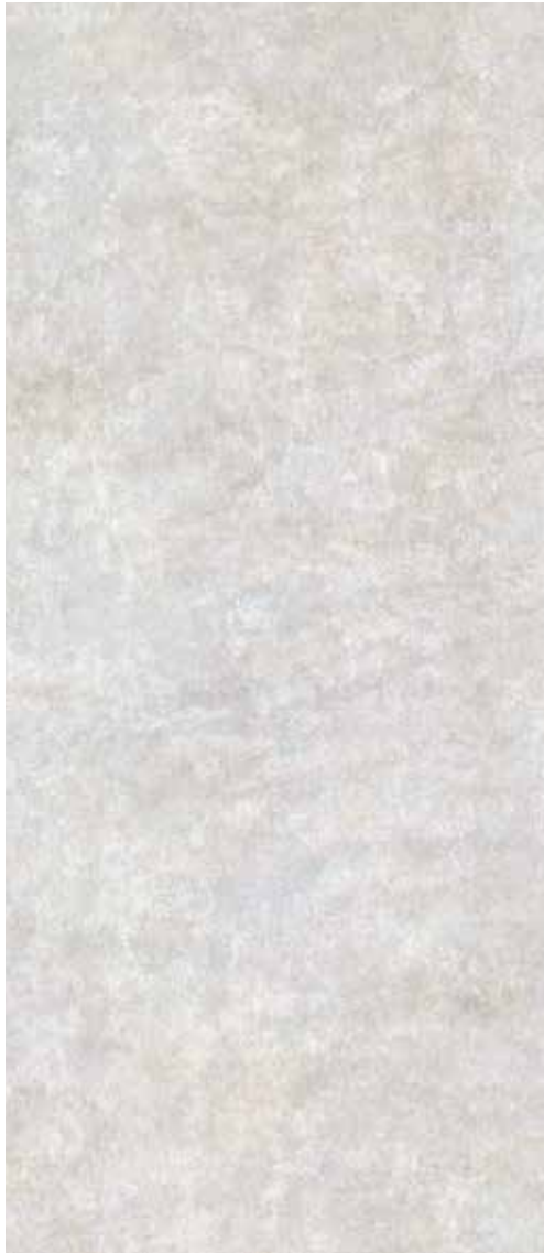
177 | stucco eroded light
